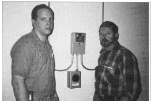
Jim Pompetti (right) of Pompetti Heating and Air and Jim Grajewski (left) maintenance supervisor for Media Real Estate, review a TMC installation.
