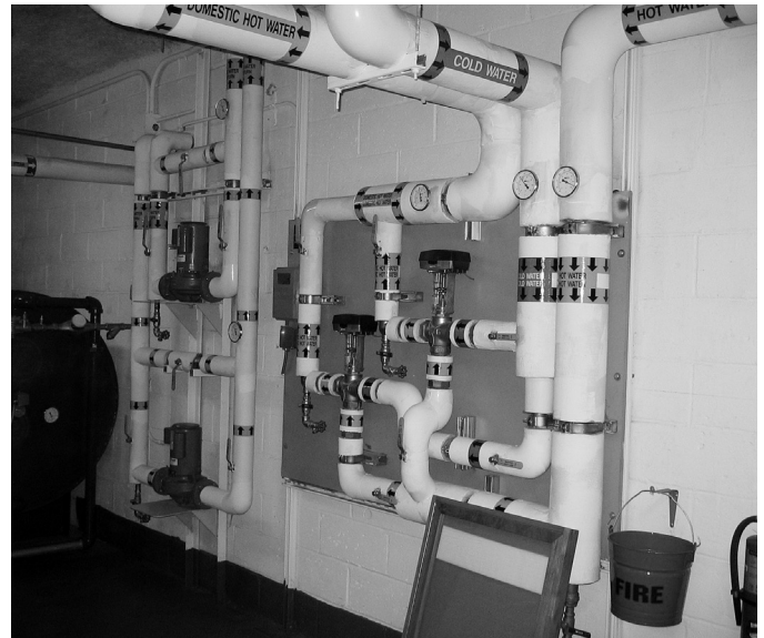
Heat-Timer ETVs (Electronic Tempering Valves) mix hot and cold water accurately to provide a safe domestic hot water temperature of 135°F at Kips Bay.
